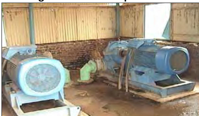
High Lift Set of Pumps
