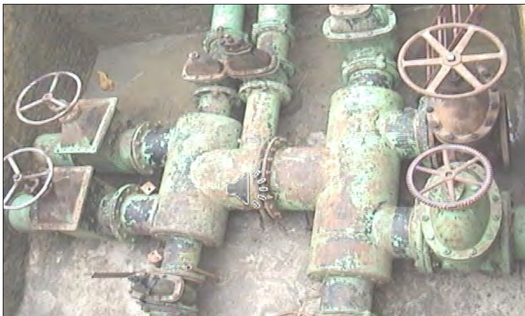
Conveyance System(Raw water)
