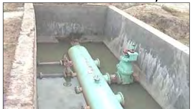
Purification Water Distribution System
