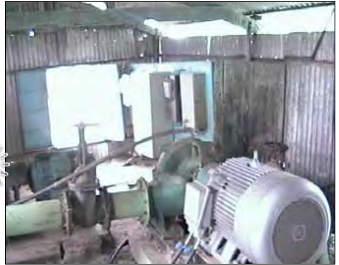
Intake No. (2), Low Lift Pumps
