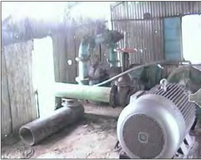
Intake No. (1), Low Lift Pumps
