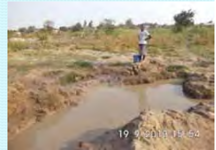
Vandalized TAZARA Rising Main – Chitulika, Mpika District
